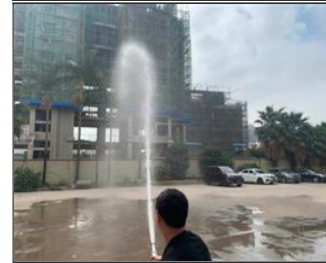
External photo(s) of the production unit(s) Testing of fire hydrant.JPG
